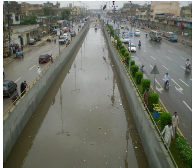
Photo 2: The newly constructed underpass looks like a lake during torrential rain
